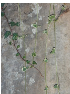
English Ivy and Blue Periwinkle continue to claim the limestone at Jenolan, covering 430 million-year-old marine fossils; sending roots into the cracks; and splitting the rock in the natural environment and in early European landscaping.
